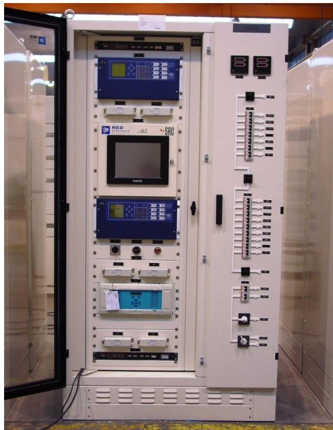
An example of one utilities' standardised protection and control bay
